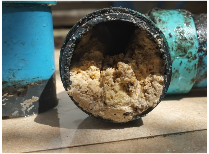
Fats, oils and grease clogging pipes
