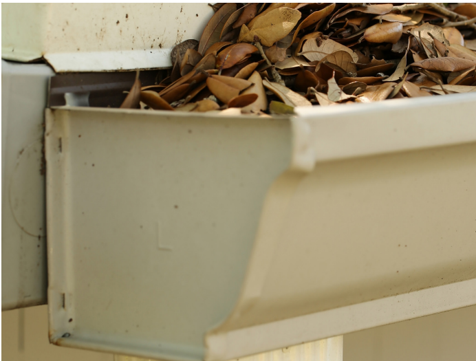
Debris from gutters or cleanouts filling pipes
