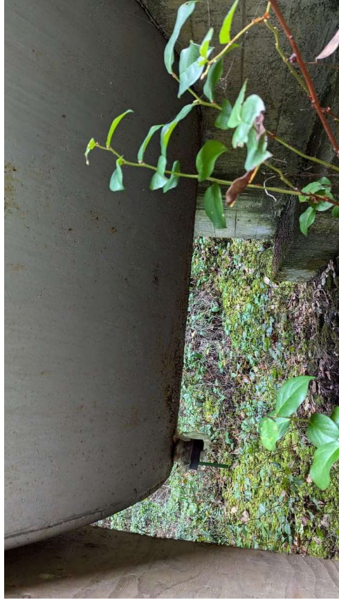
Figure B-8 Exterior Base of Tank 2
