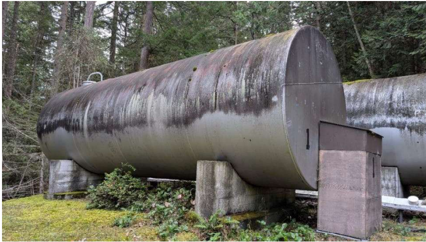
Figure 2-2 Skana Water Storage Tanks
