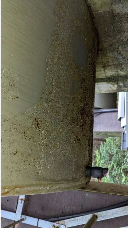
Figure B-2 Exterior Base of Tank 1
