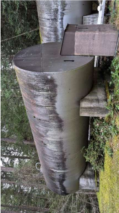
Figure B-1 Tank
