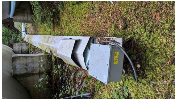
Figure B-3 Raceway Between Tanks
