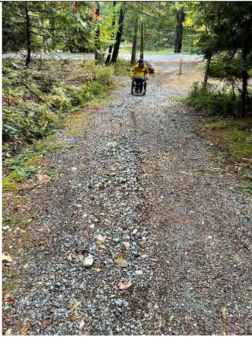
Erosion Channels in Steeper Segments of Trail Expose Base Materials and Create Barriers
