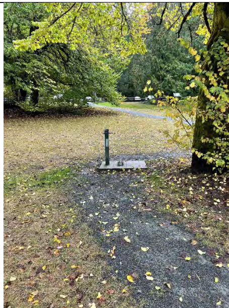
Inaccessible Potable Water – Access & Tap Function
