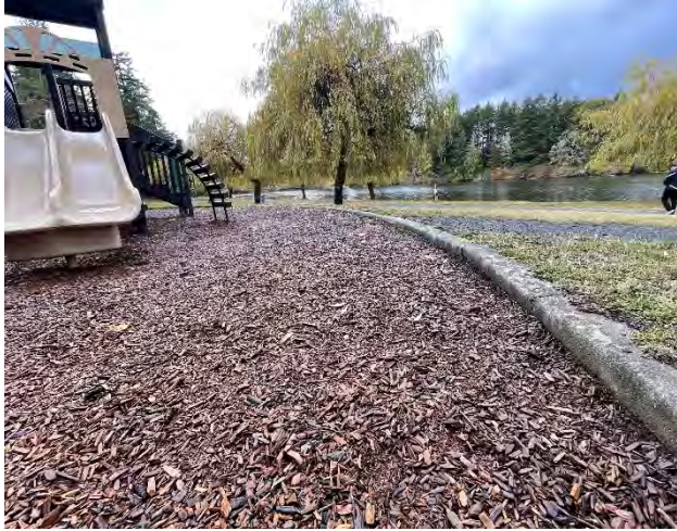
Inaccessible Playground – Surfacing & Significant Concrete Transition
