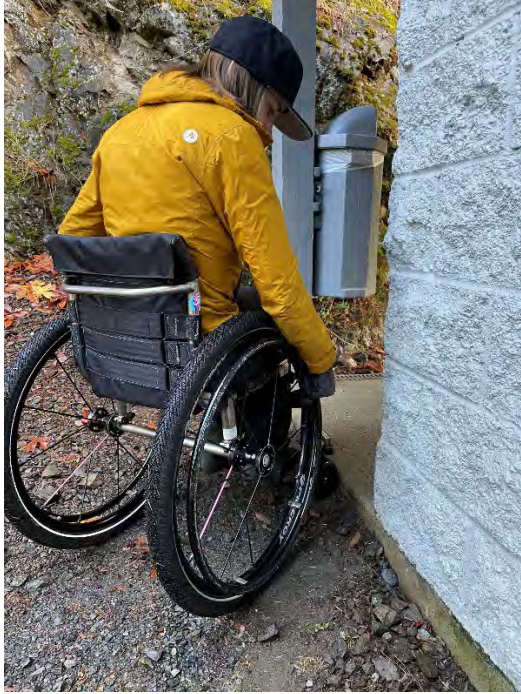
Transition into the Toilet Building is a Barrier
