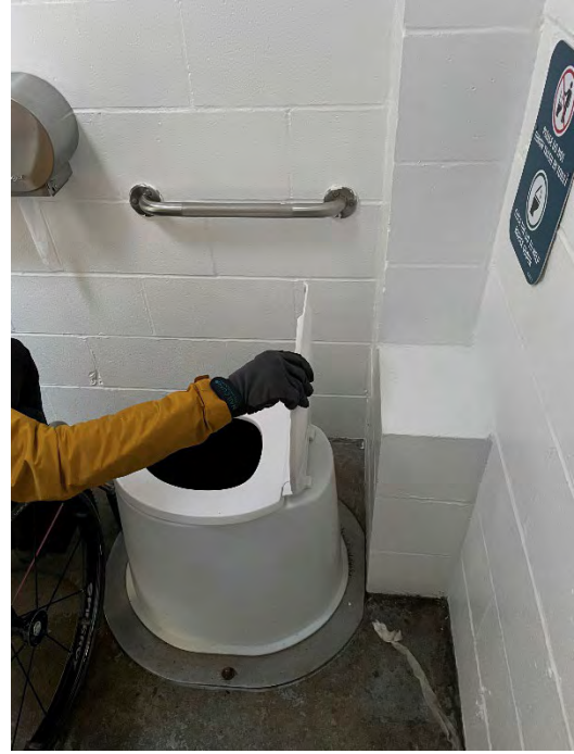
Gap Between Toilet Throne and Back Wall Does Not Support People with Limited or No Core Strength and Poses a Risk for Falling Off the Toilet
