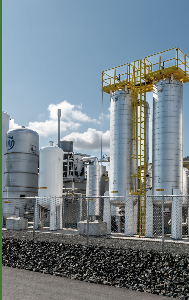
RNG Facility, Hartland Landfill
