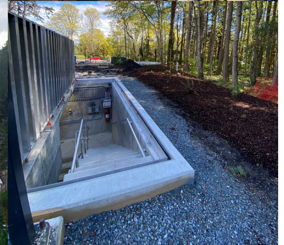
Arbutus Attenuation Tank
