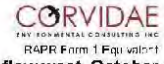
Photo 3. Culvert under Powder Main Rd where ditch and neighbour's stream join and flow west. October 2020.
