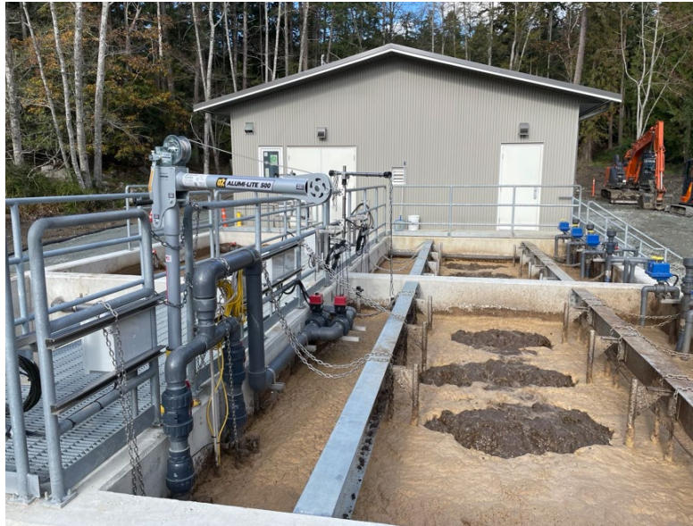
Schooner WWTP in Operation
