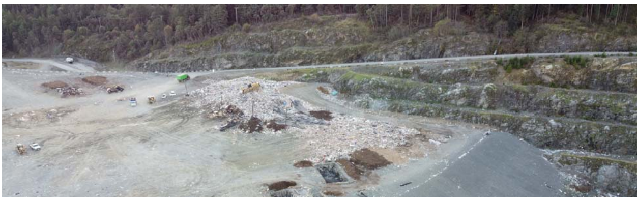
Photo 4.6 - Waste Disposal at West of C1 area Over the Rock Wall Area, October 2020
