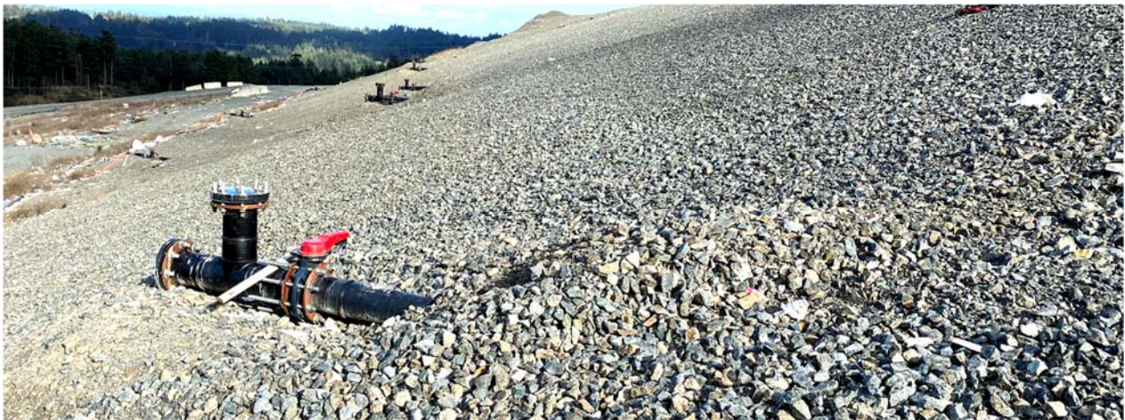
Photo 4.7 - New Horizontal Collectors (Area S14)
