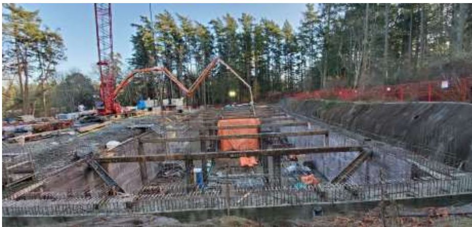
Figure 13 – Arbutus Attenuation Tank- Attenuation Tank Overview.
